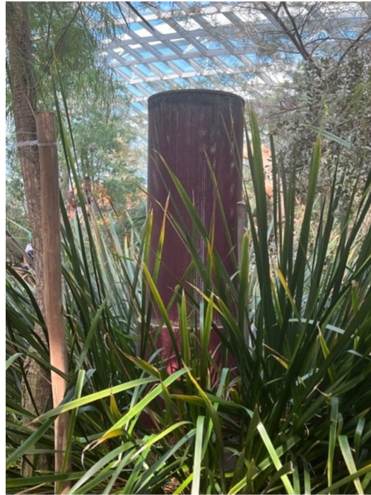
Figure 17: Air diffusers introduce cold air to the lower, inhabited parts of Flower Dome. Photo: Nadine Chan.
