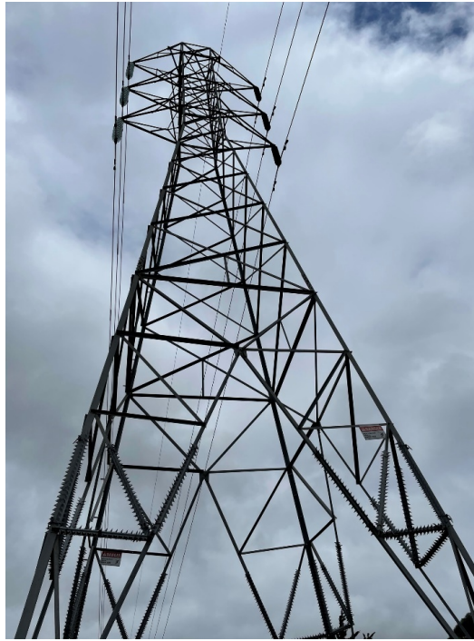
Figure 1: An electricity tower in PG&E's service territory, just outside San Luis Obispo, California.
